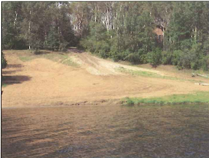
PHOTO 3 Eroded slope at Cabin1 Area.
