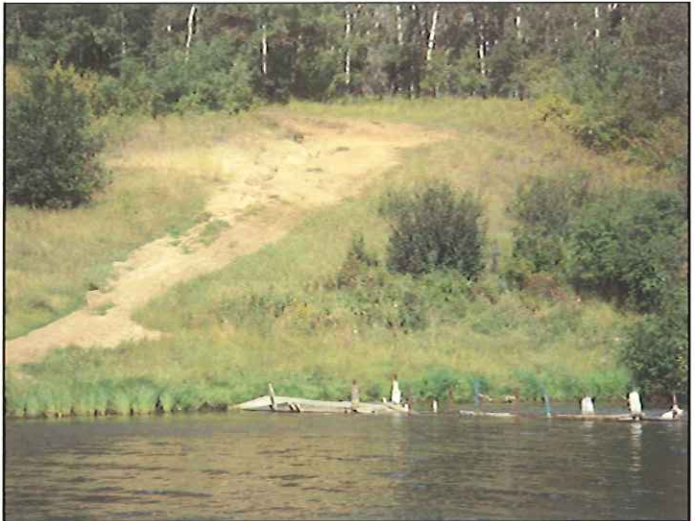
PHOTO 4 Eroded slope at Cabin1 Area.
